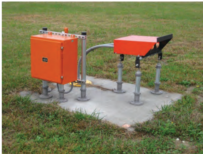
Figure 4.6. PAPI unit. Source: Delta Airport Consultants, Inc.
