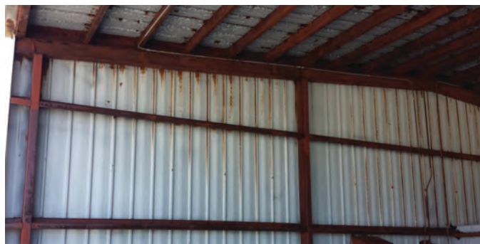
Figure 2.2. Rusted hangar not usable for aircraft storage. Source: Delta Airport Consultants, Inc.
