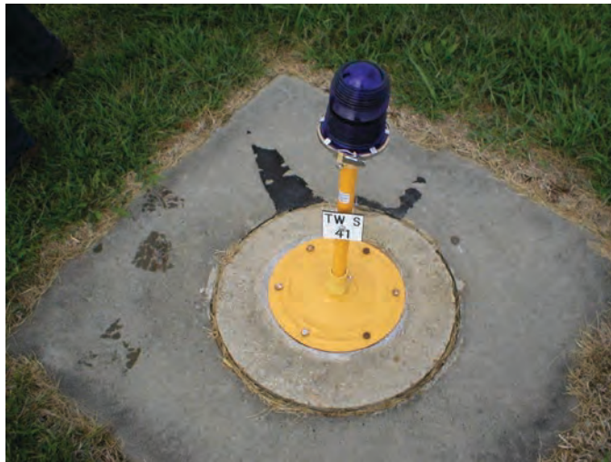
Figure 4.2. Taxiway edge light. Source: Delta Airport Consultants, Inc.
