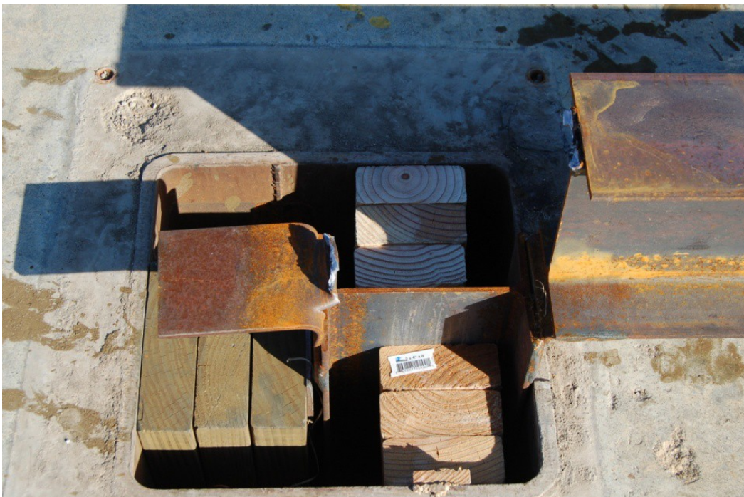
Figure 5: Welded tab post after test (TEST SDCB-1).
