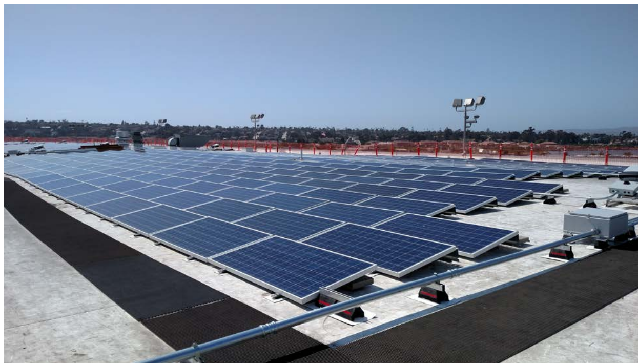
Figure 7-5. Solar PV on the Roof of Terminal 2 at San Diego Airport
