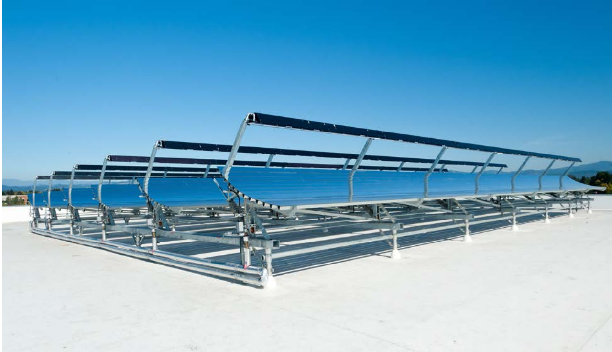
Figure 7-1. Hybrid Solar Installation at Facebook's Menlo Park Campus
