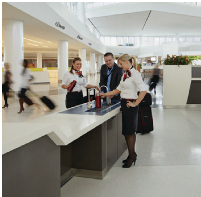
Figure 8-4. Hydration station, San Francisco International Airport Terminal 2.
