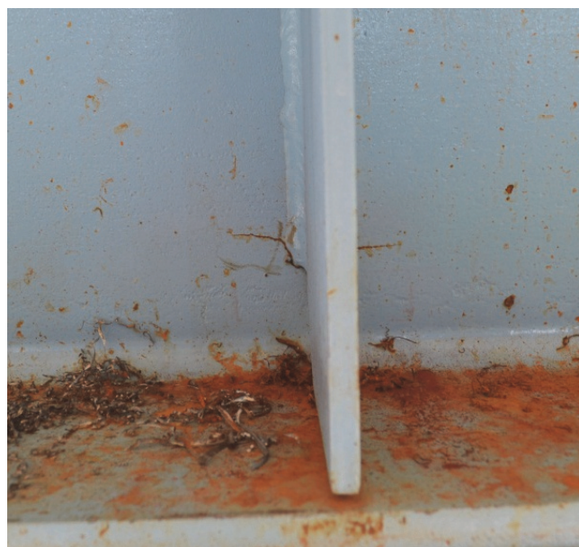
FIGURE 2 Out-of-plane and distortion-induced cracking (Snyder 2015).
