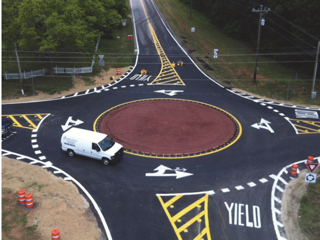
FIGURE 36 Accelerated low-cost roundabout installation at the intersection of SR-11/SR-124/Galilee Church Road in Jackson County, Georgia. Source: Zehngraff (50).
