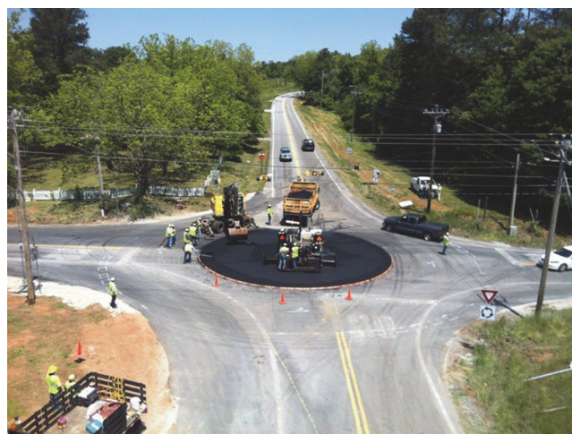
FIGURE 35 Intersection of SR-11/SR-124/Galilee Church Road in Jackson County, Georgia, during second weekend of construction of the accelerated low-cost roundabout. Source: Zehngraff (50).
