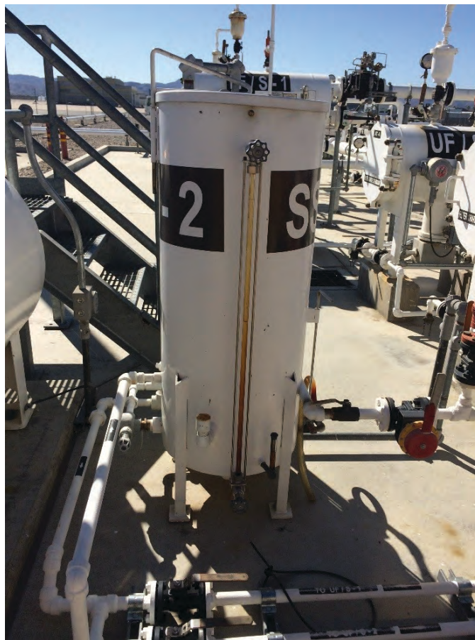
FIGURE 19 Sump recovery tank (Source: L. Valle 2015).
