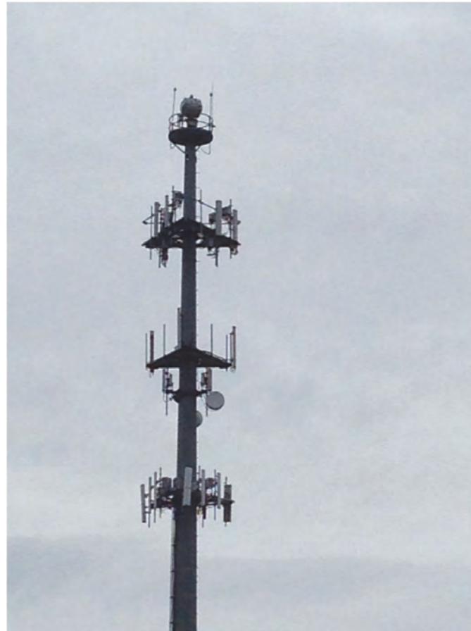
FIGURE 11 Rotating beacon atop cell phone tower (Source: J. Black 2015).
