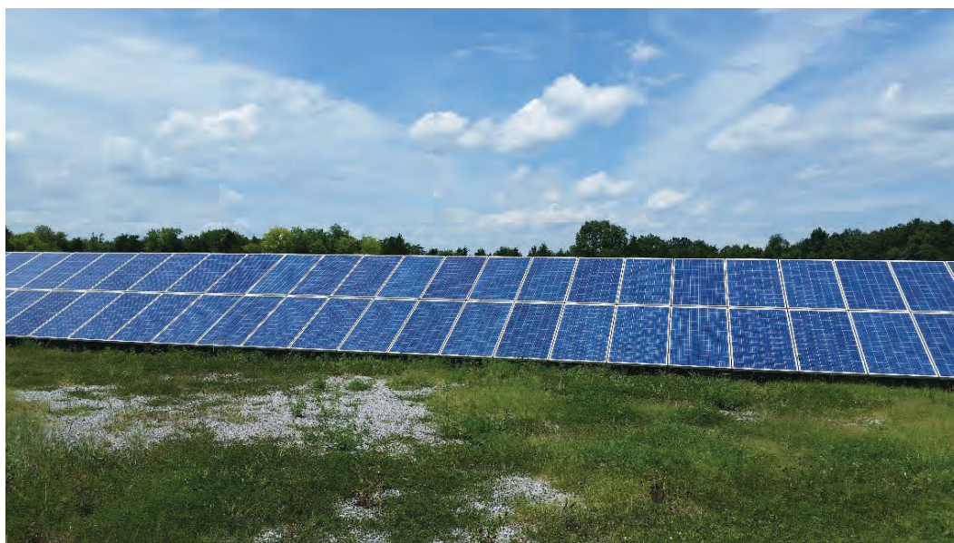
FIGURE 10 Smyrna/Rutherford County Airport PV solar field (Source: D. Prather 2016).
