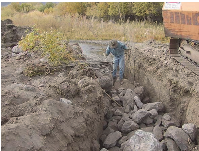
Figure 4.25. Construction of keys provides an opportunity for deep planting willow poles (McCullah and Gray 2005).
