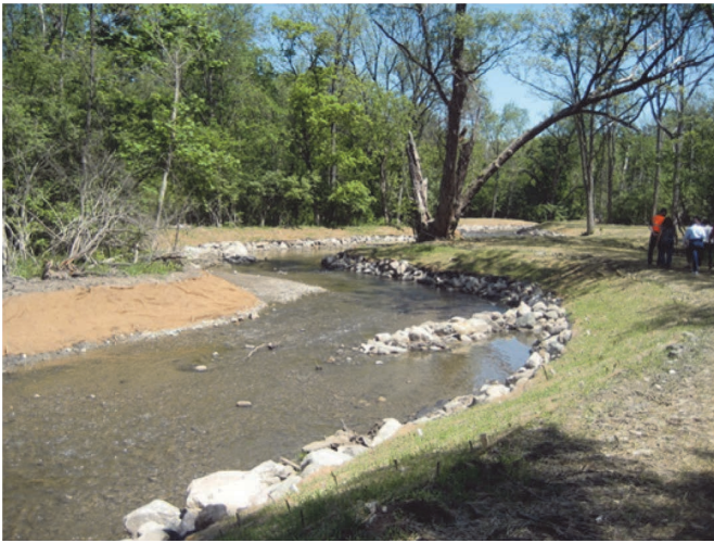
a. Graded bank, stone toe, and upstream-angled rock vane shortly after construction.
