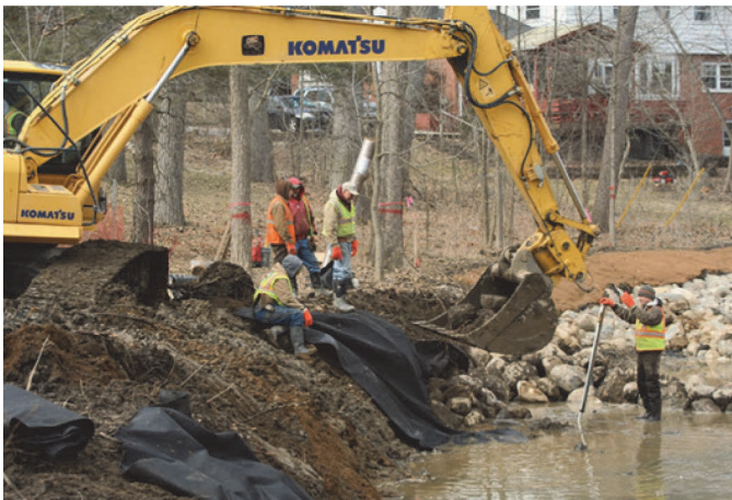
i. Construction crew installing filter fabric on graded bank prior to placing stone. Permission from OHM, Inc.
