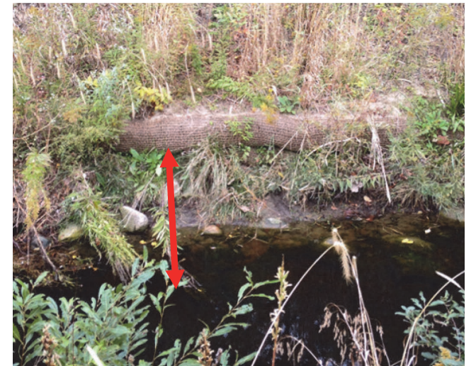
f. Close-up view of channel bank with coir log toe two years after construction. Red arrow indicates about 1.5 ft of bed degradation.
