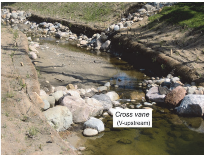
c. Graded bank with coir logs at toe and stone cross vane shortly after construction.
