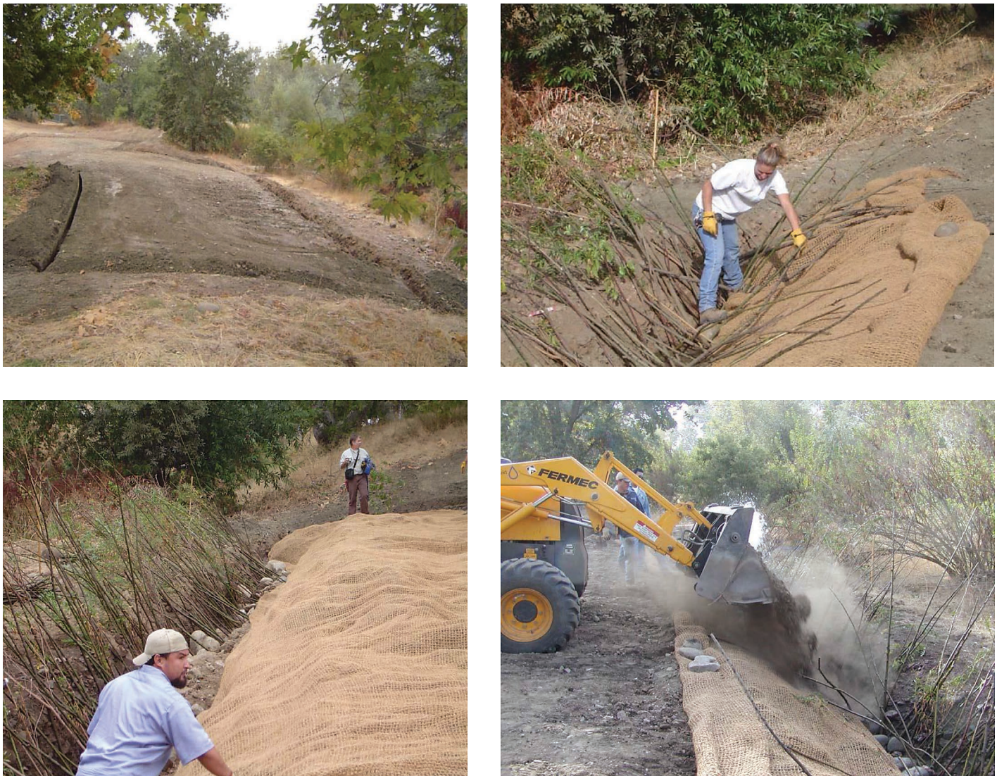
Figure 4.23. Construction and installation of live siltation on Alamitos Creek, CA (McCullah and Gray 2005).
