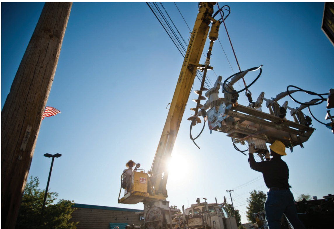
FIGURE 4-18 Installation of an IntelliRupter Pulse Closer. SOURCE: McCarthy, 2015. Image courtesy of POWERGRID International.
