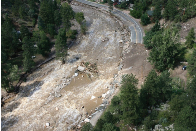
FIGURE 36 US-34 damage at MP 76.73 (Courtesy of Colorado DOT).
