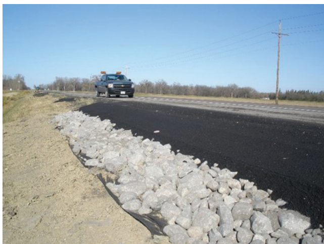
FIGURE 28 Installation of riprap placed over geotextile and then paved over (TH-9 south of Ada, Courtesy of Minnesota DOT).
