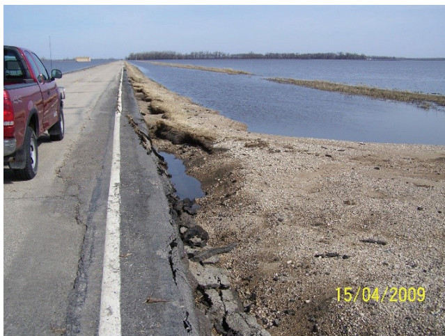
FIGURE 20 Wave damage on the downstream unprotected slope (TH-220 north of Oslo, Courtesy of Minnesota DOT).
