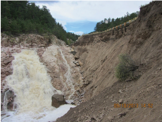
FIGURE 39 US-36 damage at MP 8.00 (Courtesy of Colorado DOT).
