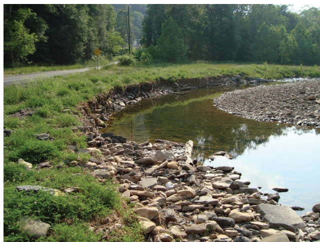
FIGURE 47 Erosion at the bend location (Courtesy of WVDOT).
