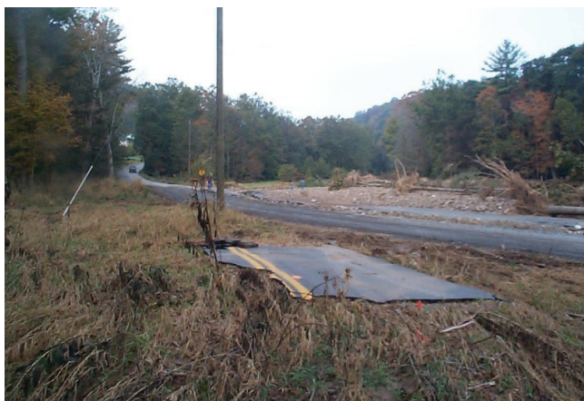
FIGURE 45 Pavement rafting after Hurricane Isabel in 2003 (Courtesy of WVDOT).
