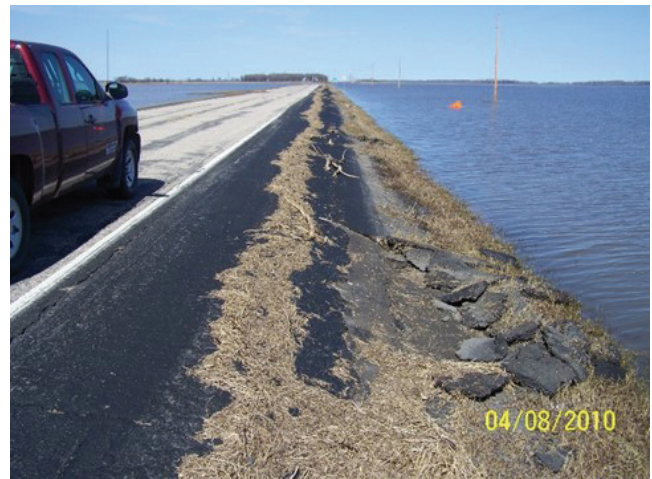
FIGURE 22 Wave damage after placing pavement on the downstream slope (TH-220 north of Oslo, Courtesy of Minnesota DOT).
