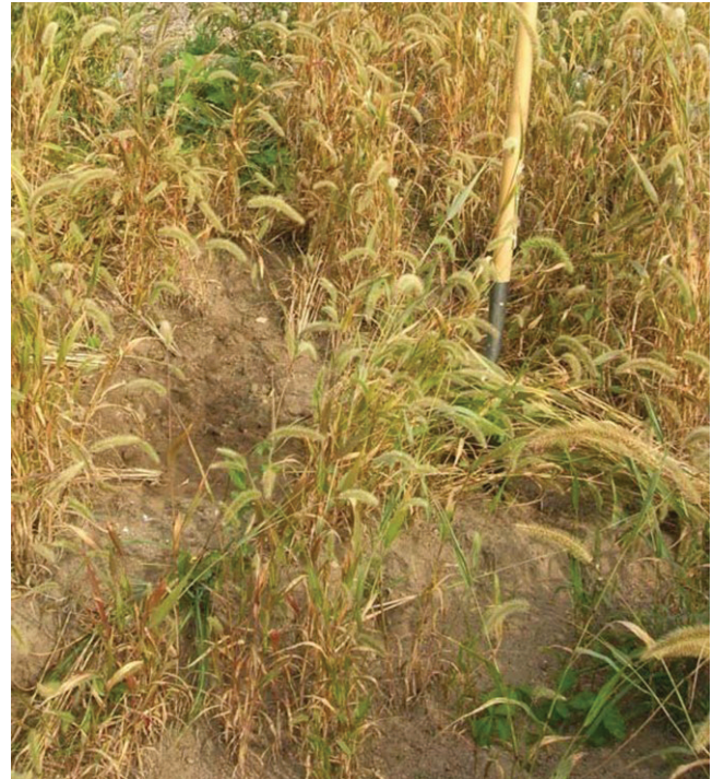
FIGURE 93 Poor-quality grass cover unable to delay erosion during overtopping (Briaud 2013).
