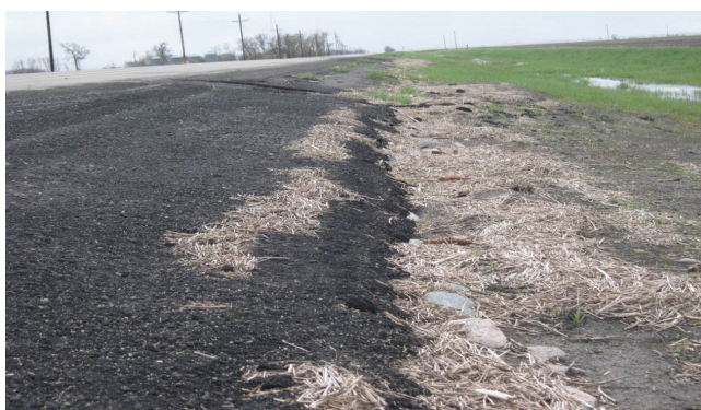
FIGURE 29 Successful performance of installed riprap system and pavement placed over it post-2011 flood (TH-9 south of Ada, Courtesy of Minnesota DOT).
