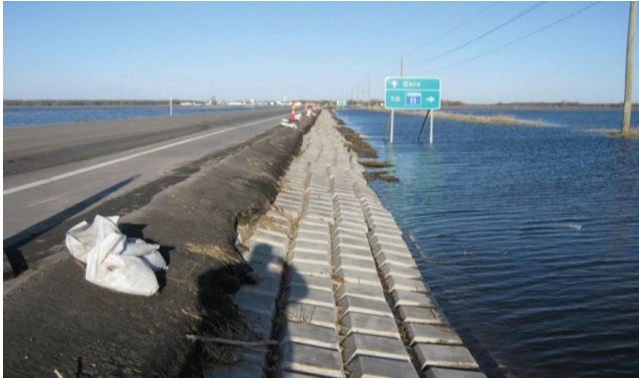
FIGURE 23 Loss of topsoil in the 2011 event after the installation of articulated concrete blocks on the downstream slope (TH-1 east of Oslo, Courtesy of Minnesota DOT).
