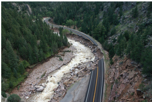
FIGURE 33 SH-7 damage at MP 27.28 (Courtesy of Colorado DOT).
