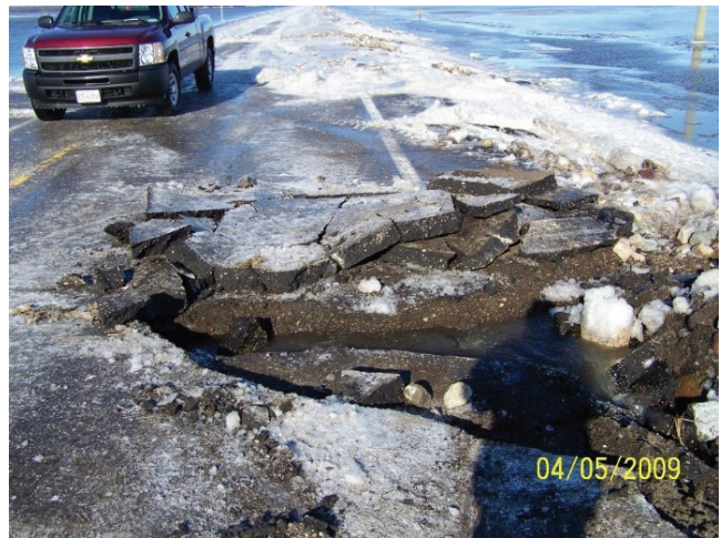
FIGURE 26 Overtopping damage in 2009 flood (TH-1 east of Oslo, Courtesy of Minnesota DOT).
