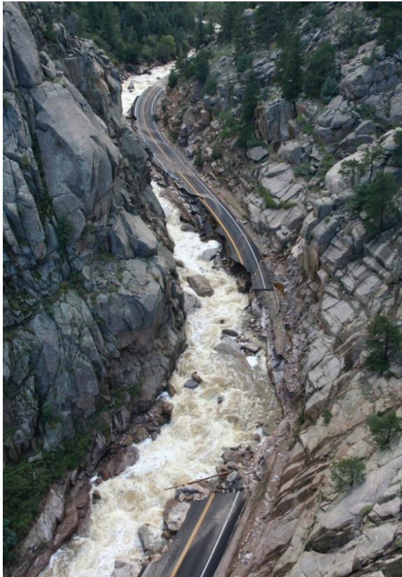
FIGURE 32 SH-7 damage at MP 27.68 (Courtesy of Colorado DOT).
