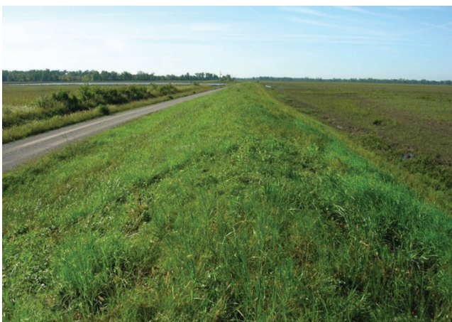
FIGURE 92 Good-quality grass cover to delay erosion during overtopping (Briaud 2013).
