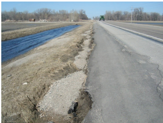
FIGURE 27 Overtopping damage in 2009 flood (TH-9 south of Ada, Courtesy of Minnesota DOT).
