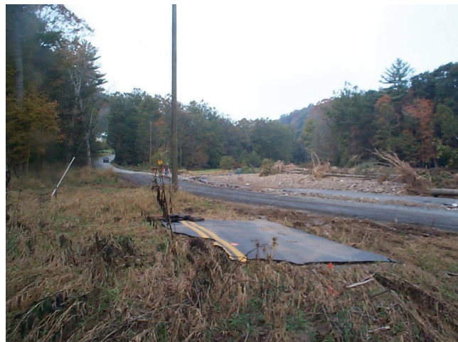
FIGURE 97 Pavement rafting damage after Hurricane Isabel in 2003, Kimsey Run Project, West Virginia.
