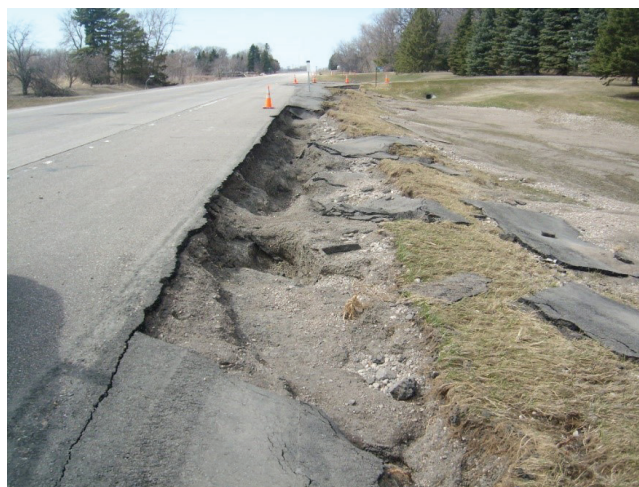
FIGURE 30 Failed downstream slopes with asphalt pavement placed on them in 2009 flood (TH-200 west of Ada, Courtesy of Minnesota DOT).
