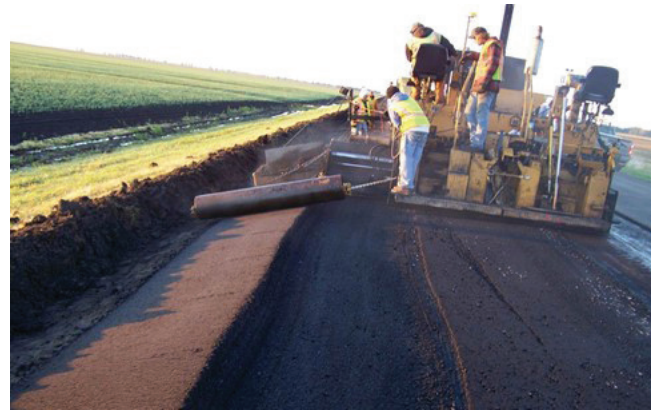
FIGURE 21 Placing pavement on the slope (TH-220 north of Oslo, Courtesy of Minnesota DOT).
