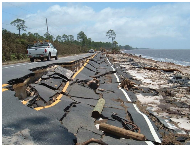
FIGURE 13 Damage from Hurricane Dennis (2005) along US-98, Franklin County, Florida (Courtesy of Florida DOT).
