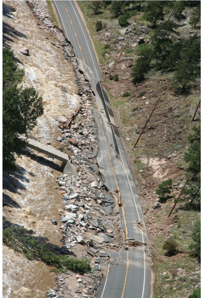
FIGURE 34 US-34 damage at MP 75.05 (Courtesy of Colorado DOT).
