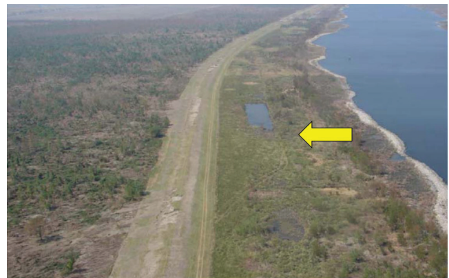
FIGURE 94 Overtopped earth embankment that survived well after 2 hours of hurricane surge overtopping (Briaud 2008).
