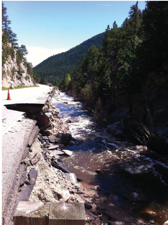
FIGURE 37 US-36 damage at MP 7.70 (Courtesy of Colorado DOT).
