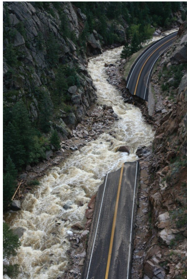
FIGURE 31 SH-7 damage at MP 26.90 (Courtesy of Colorado DOT).
