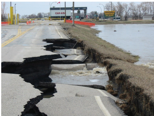
FIGURE 96 Pavement damage, washed-out culvert, and embankment breach in 2009 overtopping during spring thaw, Highway 18, North Dakota.
