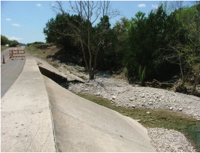
FIGURE 112 Failure of concrete lining (RM-335, Real County, Courtesy of TxDOT).
