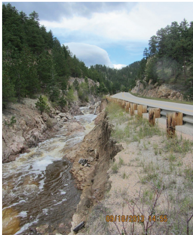
FIGURE 38 US-36 damage at MP 7.80 (Courtesy of Colorado DOT).
