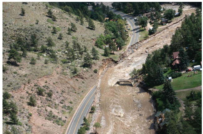
FIGURE 35 US-34 damage at MP 76.40 (Courtesy of Colorado DOT).
