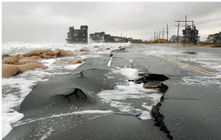
FIGURE 7 Pavement damage from surge and waves (13).
