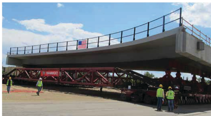
Figure 6.6. Pecos Bridge: (top) rendered view of bridge movement (Source: Kiewit), (bottom) picture of SPMTs and bridge superstructure (Source: Aspire, Winter 2014).
