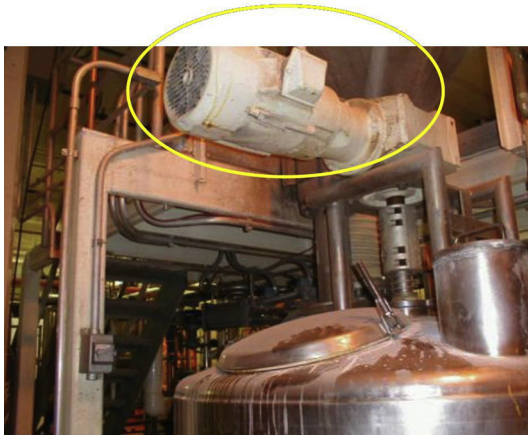
FIGURE 6.53 Drive motor is installed above the manhole of the process vessel. When the manhole cover is open, the product may become contaminated with lubricants, condensate, or dirt discharged from the drive motor ( organization Sanitary Design Workshop , © 2016).
