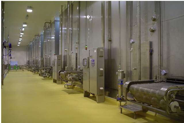
FIGURE 6.63 Sufficient distance is maintained between the cabinet base and the floor. The cabinet is positioned at a considerable distance from the wall of the enclosure. The top roof is sloped toward the front. The field boxes in smooth plastic are mounted at 45 degrees and sealed to the wall of the enclosure. Connections of cables and wires to field boxes are sealed. Courtesy of GEA Group.
