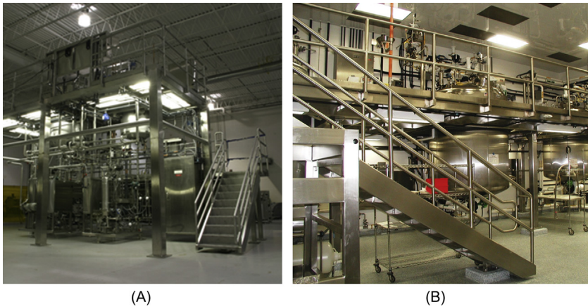
FIGURE 6.82 (A) Connecting the framework of stairs, walkways, or platforms to a floor usually occurs by means of a base plate securely fastened to the floor by means of a fixing bolt (courtesy of Holland Applied Technologies). (B) Base plates also can be fixed to a floor plinth, thus prohibiting dirt and liquids from getting under the base plate during process and cleaning operations. The stringers of staircases make no floor contact, hence facilitating the cleaning of the factory floor. Photo left, courtesy of Holland Applied Technologies; photo right, courtesy of Bay State Industrial Welding & Fabrication, Inc.)
