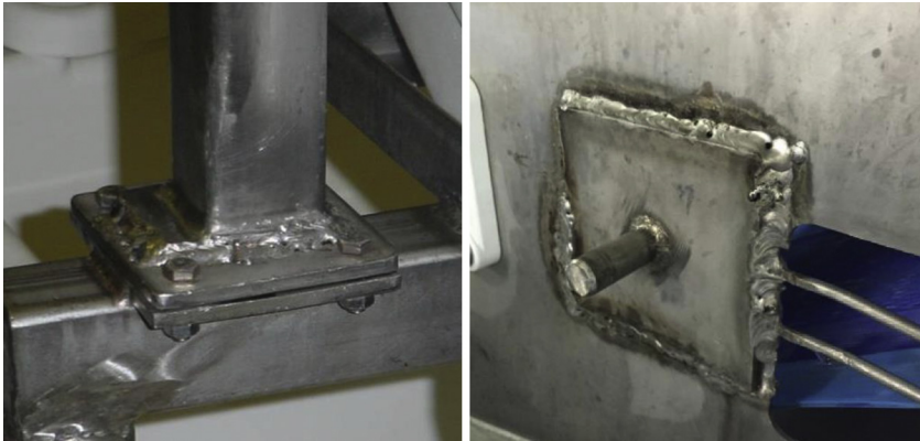
FIGURE 6.3 Welds must be continuous and smooth, free of pits and cracks. Gaps, lap seams, bolts, and threads will accumulate dirt and will make this equipment not cleanable. Photo left, courtesy of John Butts, Land O’Frost, © 2016; photo right, courtesy of Joe Stout, Commercial Food Sanitation LLC - Intralox, ©2016.
