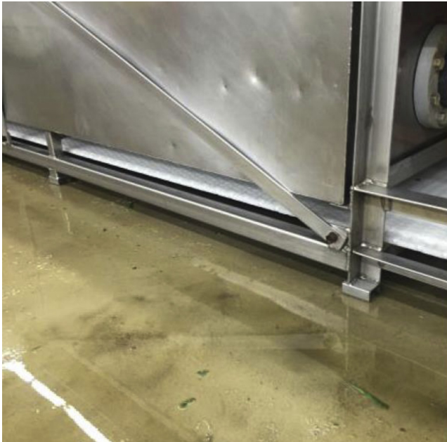
FIGURE 6.79 Process equipment should be installed as high off the ground as possible to facilitate cleaning and reduce the risk of cross-contamination during cleaning operations. In this case, dirt released from the floor during high-pressure cleaning may splash onto the process equipment. Courtesy of Joe Stout, Commercial Food Sanitation LLC - Intralox, © 2016.
