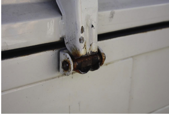
FIGURE 6.12 Paints can crack or peel off.
