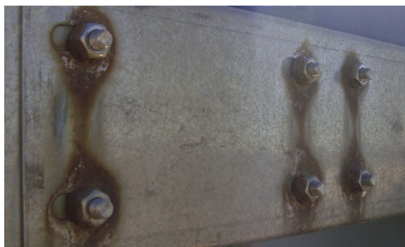
FIGURE 6.1 In this part of the food processing equipment, galvanized steel plate is combined with stainless steel bolts, giving rise to galvanic corrosion between the stainless and galvanized steel components.
