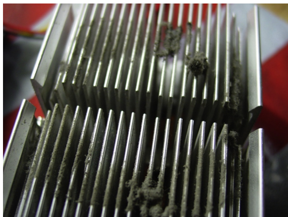
FIGURE 6.61 A cooling device that ventilates the heat produced by electrical equipment to the outside concomitantly accumulates dust and dustborne microorganisms inside the electrical equipment. Moisture- and dust-tight casings with high IP rating will reduce inside buildup of dirt, and therefore are especially recommended in dry material handling areas with high dust loads. Regular cleaning of the interior of electrical devices by vacuum is also a suitable option, but blowing with compressed air even in the presence of a dust extraction system is not recommended (Moerman, 2011).
