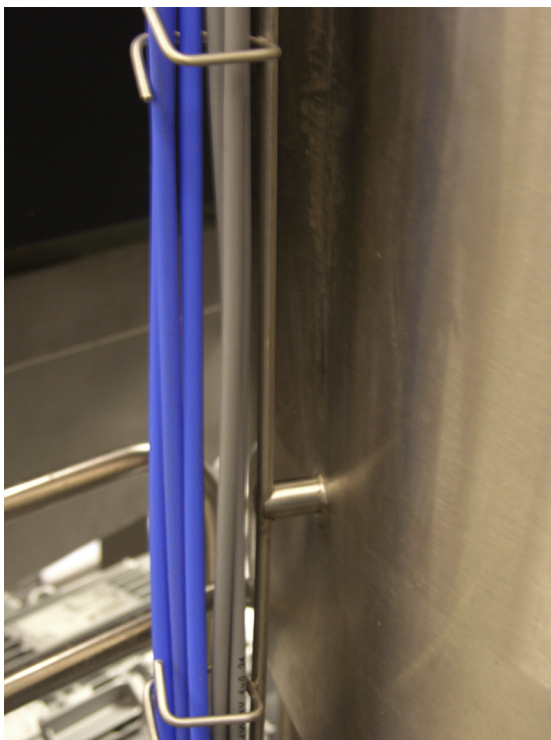
FIGURE 6.73 Cable support system with a minimum number of members. The number of loosely fixed cables should be minimal, to avoid uncleanable entangled cable arrangements.
