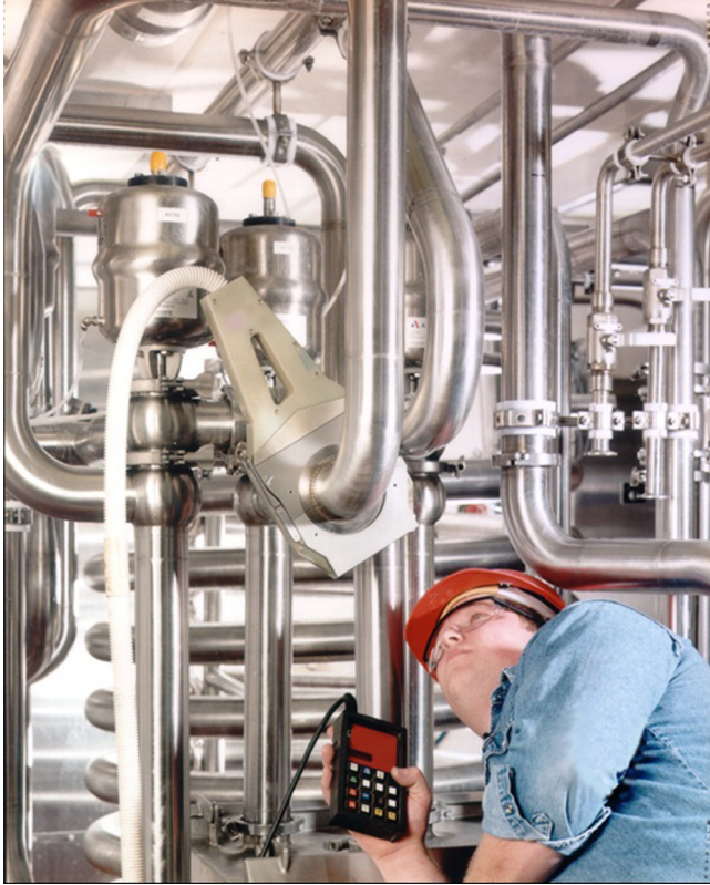
FIGURE 7.35 Stainless steel hygienic tubing joints should be made by automatic orbital welding where possible. Orbital welding provides smooth and crevice-free junctions (Kopitzke et al., 2006).
