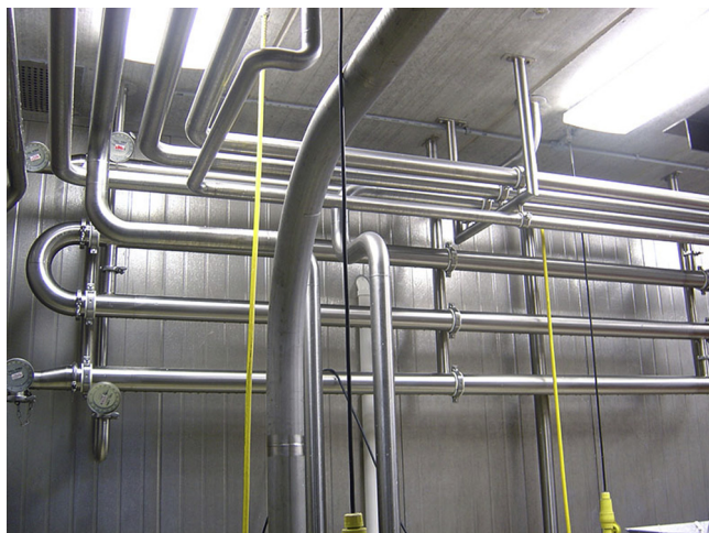
FIGURE 7.39 For suitable cleaning, process equipment and piping must be installed at sufficient distance off the wall, ceiling, and floor. Courtesy of CSI Central States Industrial, www.csi-designs.com .
