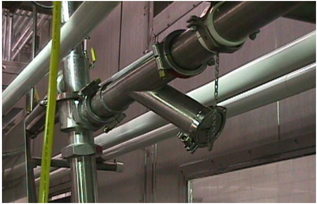
FIGURE 7.30 This drain point pointing downwards acts as a dead leg (organization Sanitary Design Workshop, © 2016).
