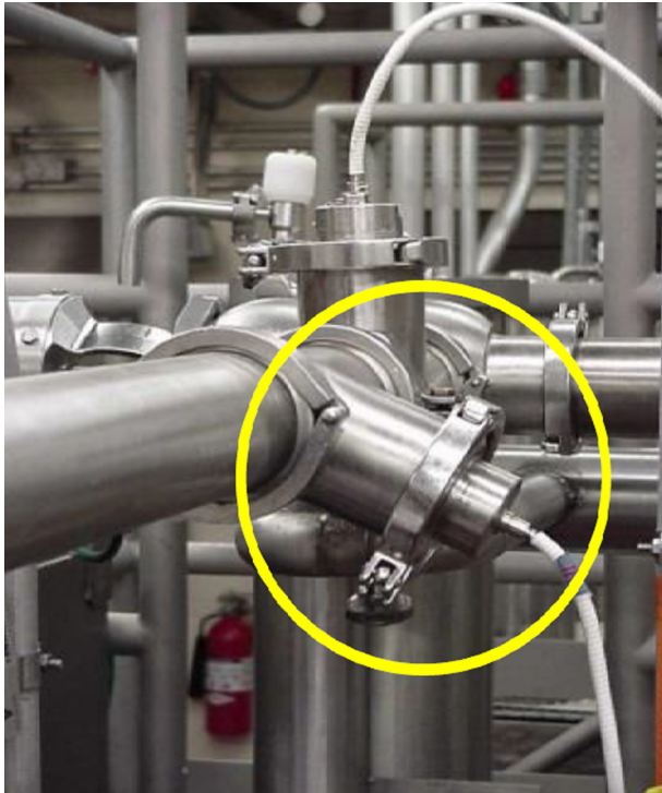
FIGURE 7.79 An instrument branch facing downward instead of inclined upwards creates a difficult-to-clean dead area where condensate, debris, suspended solid particles, flakes, etc. may accumulate. Fluid velocities in the dead leg are much lower, and thus the area of entrapment may not be reached by cleaning or sterilizing procedures, hence leading to contamination of the product. Courtesy of Joe Stout, Commercial Food Sanitation LLC - Intralox, © 2016.
