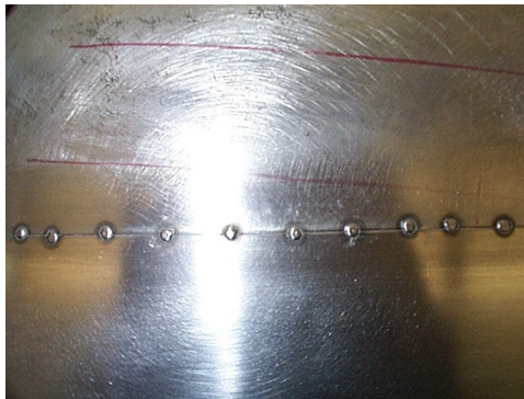
FIGURE 7.2 Spot welds create crevices and may retain product residues, as well as harbor microorganisms.
