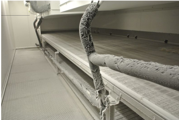
FIGURE 7.37 The cladding which surrounded the insulation of the refrigerant supply and removal piping was probably lost during high-pressure cleaning operations. Now, worn off particles of insulation may be entrained by the airflow into the product (Moerman & Fikiin, 2016).
