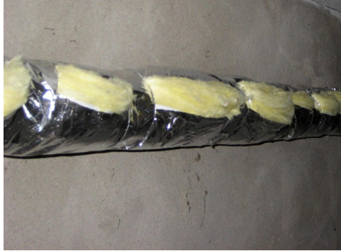
FIGURE 7.36 Fiberglass batting has been proven to be an excellent harborage of dust, insects and rodents (Moerman & Wouters, 2015).
