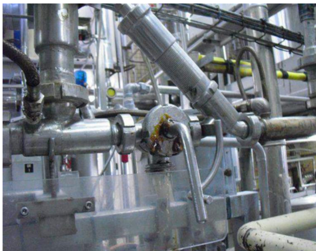
FIGURE 7.64 With respect to plug cock valves, product can get caught as a thin stagnant film around the clearance between the plug and the valve body during rotation of the plug, and finally may leak to the outside. Courtesy of Mondelez International, © 2016.
