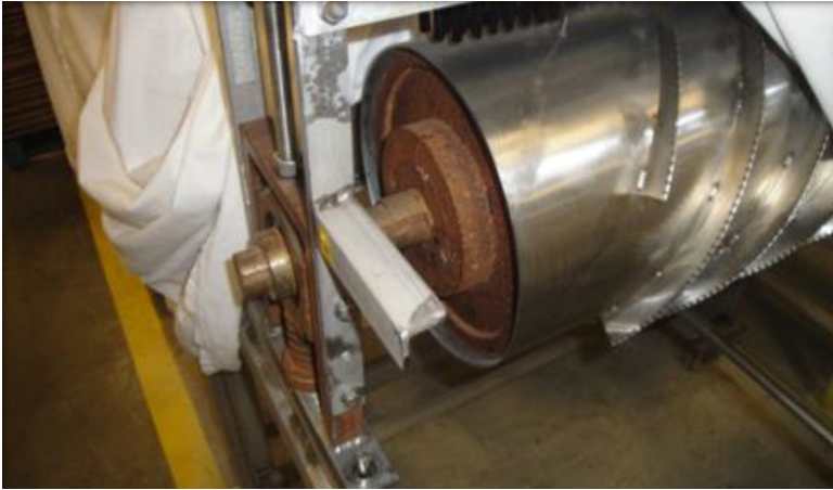
FIGURE 8.14 Stainless-steel shell and knives of the roller are combined with roller ends in mild steel. As mild steel is less noble than stainless steel, it will corrode. Work in black steel and stainless steel must always be kept separate. Courtesy of organization Sanitary Design Workshop, © 2016.
