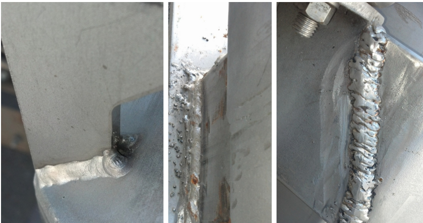
FIGURE 8.18 Poor weld repair. Courtesy of Rudi Groppe, Heinzen Manufacturing International, © 2016.
