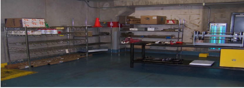
FIGURE 8.49 Storage room for replacement parts, maintenance tools and maintenance aids should be neat and clean, and allow storage in dry conditions. Courtesy of Mondelez International, © 2016.
