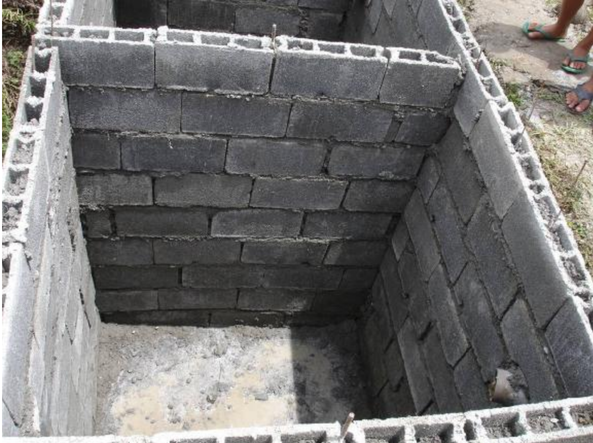
Figure 9 - GK Nazareno (Samal Island, Mindanao) with open bottom single chamber septic tank.
