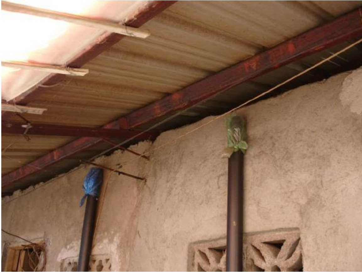
Figure 10 - GK Assumption (Batangas). Note the covered exhaust pipes extending to just below the roofline.
