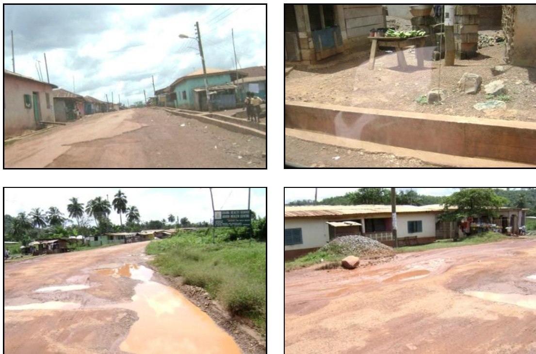
Figure 4.4: Road conditions on the way to the Damang mine site
