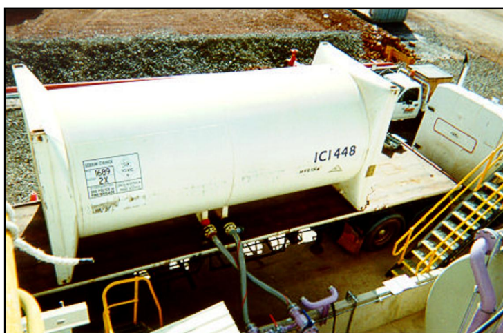
Figure 2.6: Sparge iso-tanker offloading at a site (OTM, n.d.)
