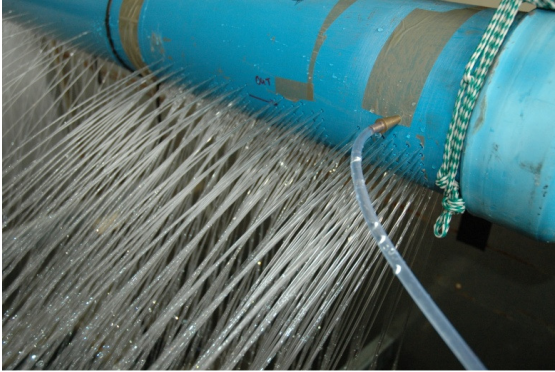
Figure 5.17: Pipe spray nozzle in operation
