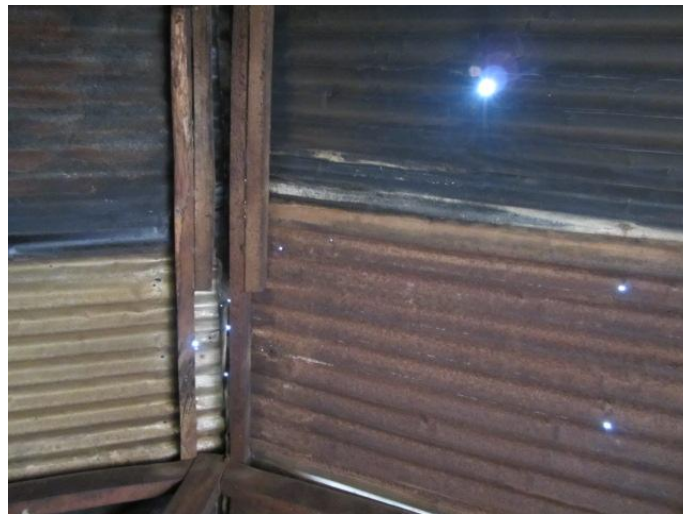
Figure 4. Holes in the roof of an informants' home. Photo: Solange Berleen Musoke, 2011
