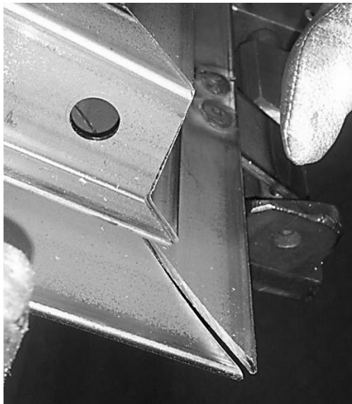
Figure 9: Gaps between steel profiles
