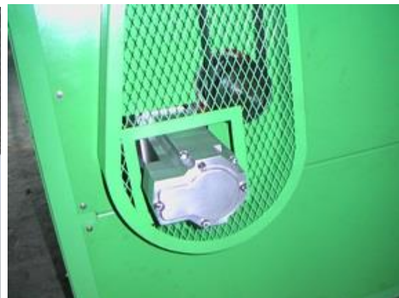
Figure 3.1.11 Pulley assembly to gearbox
