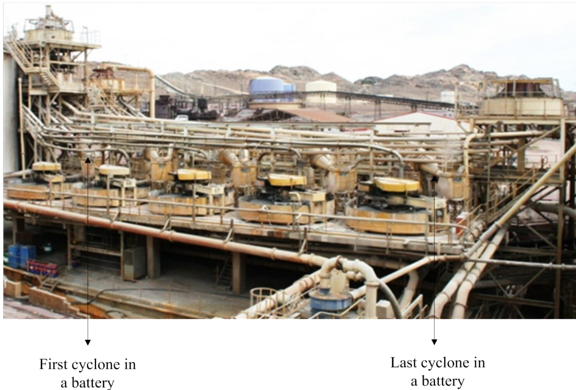
Figure 4-4: RUL hydrocyclones plant/circuit layout indicating the first and last cyclone in a sequence
