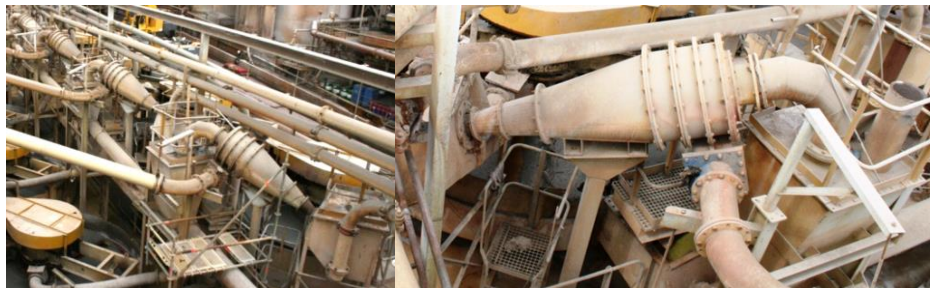
Figure 4-7: RUL hydrocyclones in a sequence as well as a zoomed-in individual cyclone
