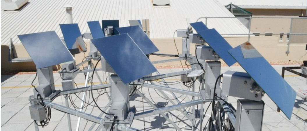
Figure 5.6: Heliostats deployed on triangular 'six-pack' pedestals.
