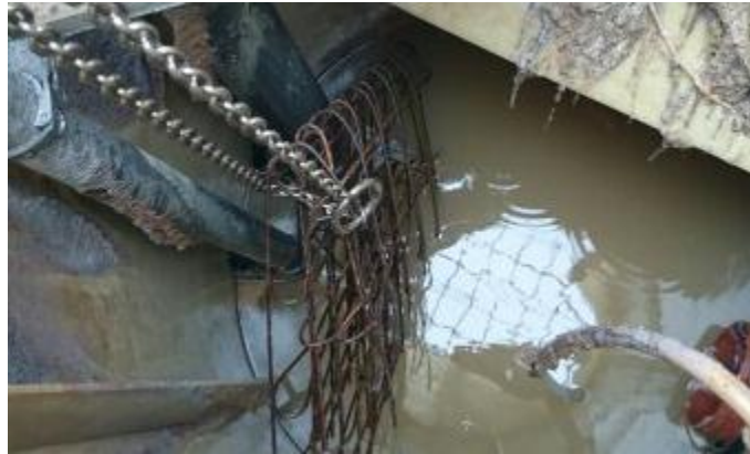
Figure 25. The sacrificial anode inside Odomin.
