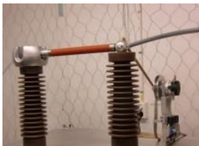
Figure 3.2: Automatic ground and high-voltage resistor 100 MΩ
