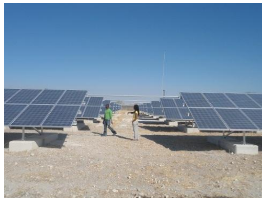
Figure 8: The solar field of the Tsumkwe Hybrid Solar-Diesel power station
