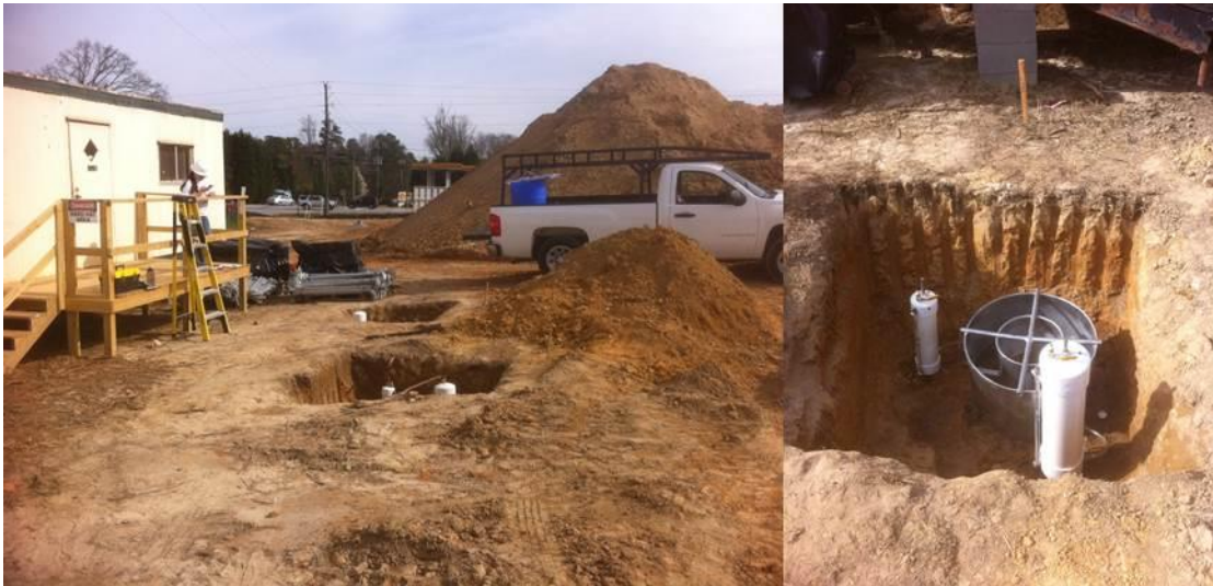
Figure 3-3 Two test pits located at the Lawrenceville, GA site are shown. A test set up is also shown in one of the test pits
