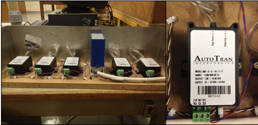
Figure B.6: 3-Fan facility pressure transducers
