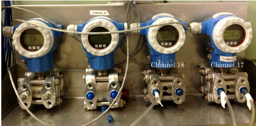
Figure B.3: Pressure transducers
