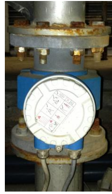
(b) Electromagnetic flow meter
