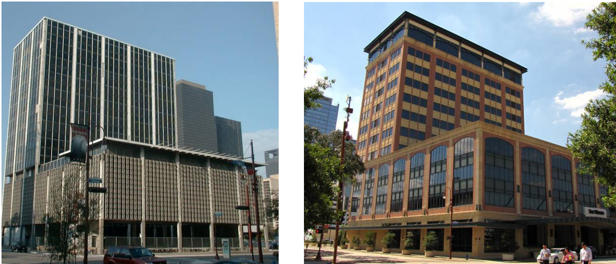
Fig.2.14. The World Trade Center (above) was vacant for several years and the curtain wall was in a bad state. Water had infiltrated and had caused severe damage. The tiles on the podium had also deteriorated and the building was completely re-skinned. It was rehabilitated to a hotel and has recently been bought by Westin.
