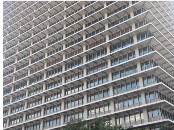
Fig.2.11. The ExxonMobil Building had marble cladding on the columns, which had deteriorated. The marble was replaced with Aluminum panels as that was easier to finish than stone.
