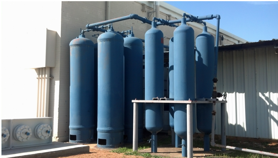
Figure 2.3: High Pressure Storage Tanks
