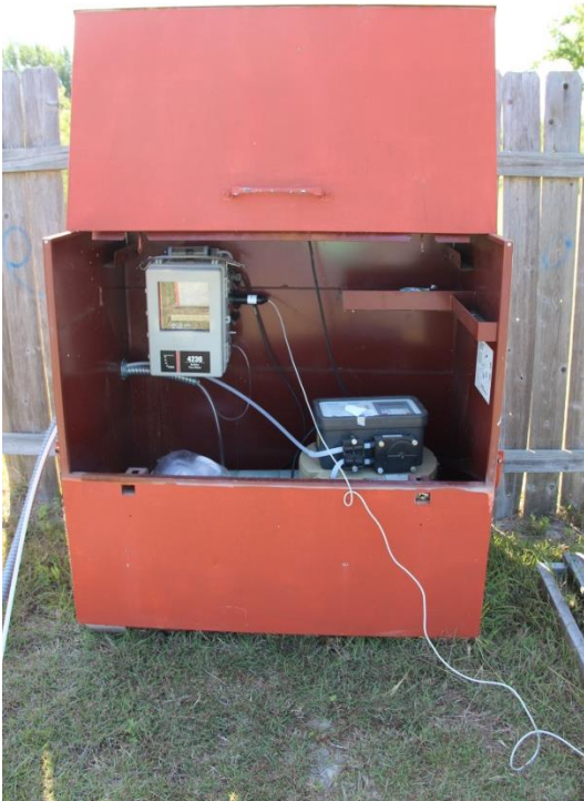
Figure 9. Water Quality Monitoring Equipment at Pon Court Basin Outlet.
