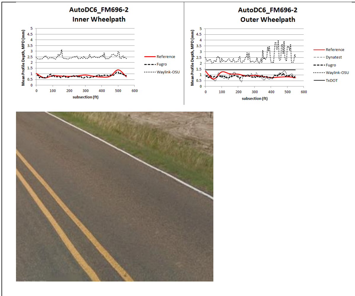
Figure A6: Inner and outer wheelpath texture graphs for AutoDC6_FM696-2 with image close-up of the pavement section
