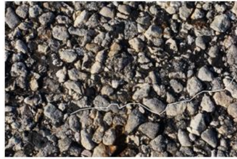
Figure 3.33: Phantom cracks marked in white (FM 1063)
