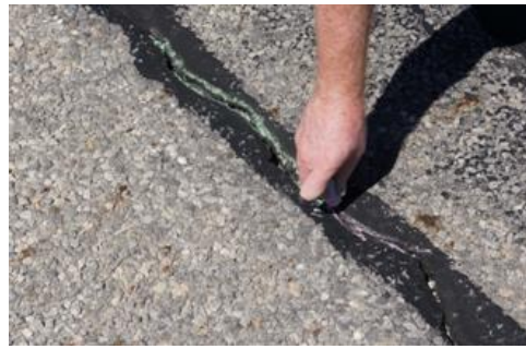
Figure 3.35: Cracks within sealed cracks (FM 1331).
