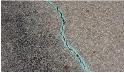
Figure 3.32: Crack marked in green (FM 1331)
