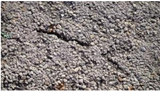
Figure 3.34: Phantom cracks created by loss of aggregates (FM 1063)
