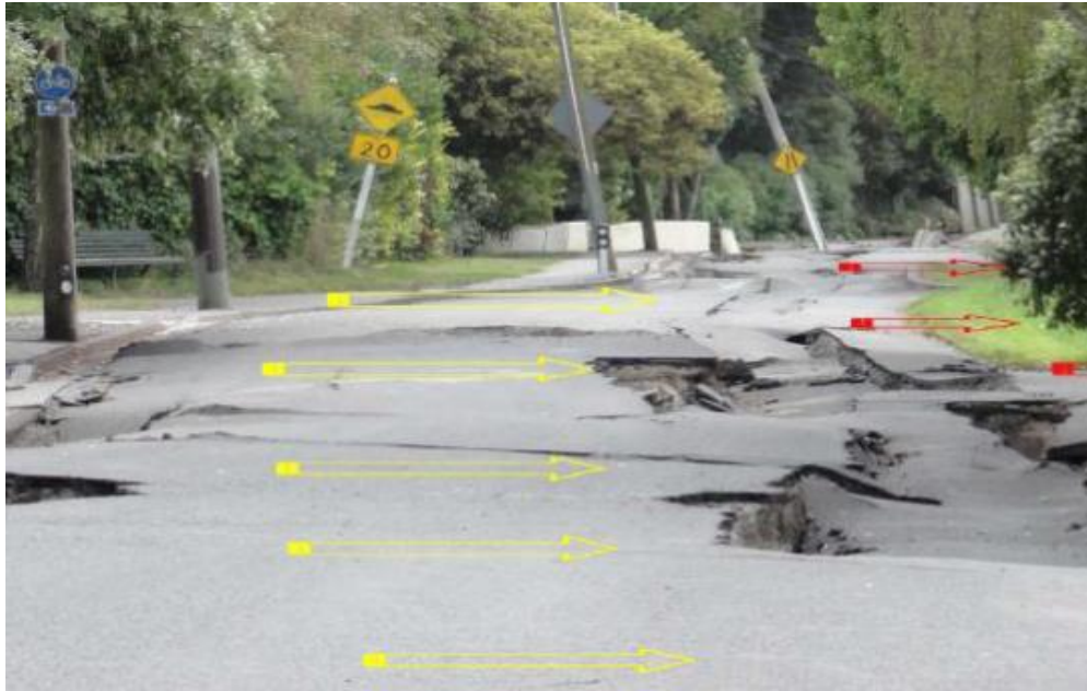
Figure 3.2. Lateral spread toward Avon River in Christchurch, NZ (Cubrinovski et al. 2011).
