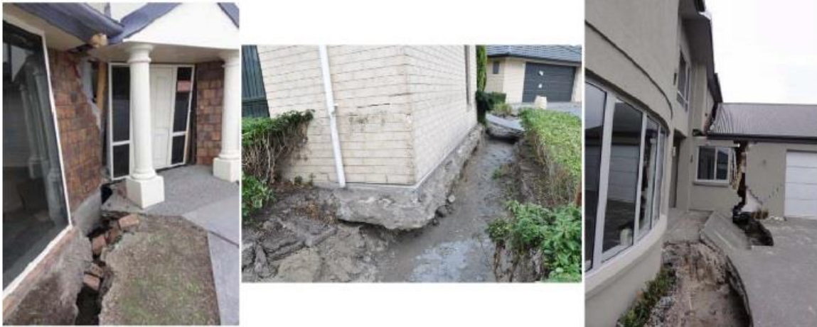
Figure 4.2. Liquefaction and lateral spreading damage in Kaiapoi, NZ (Green et al. 2010).
