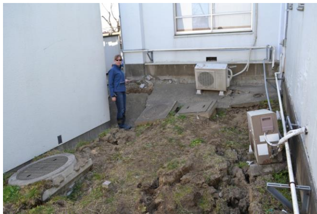
Figure 5.2. Photos showing damage from lateral spreading in Katori, Japan (Ashford et al. 2011).
