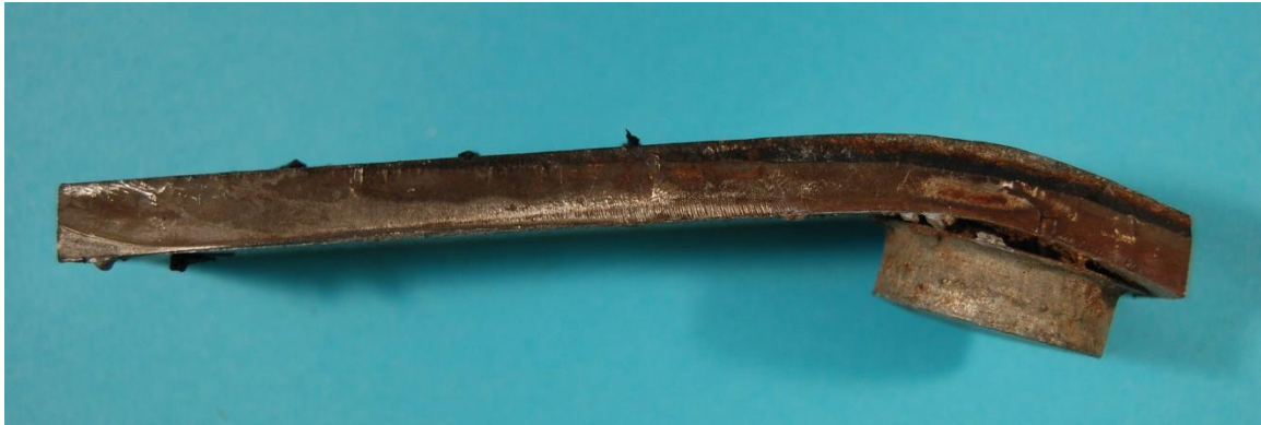
Figure 4.25: Close up of crack at Bend 8
