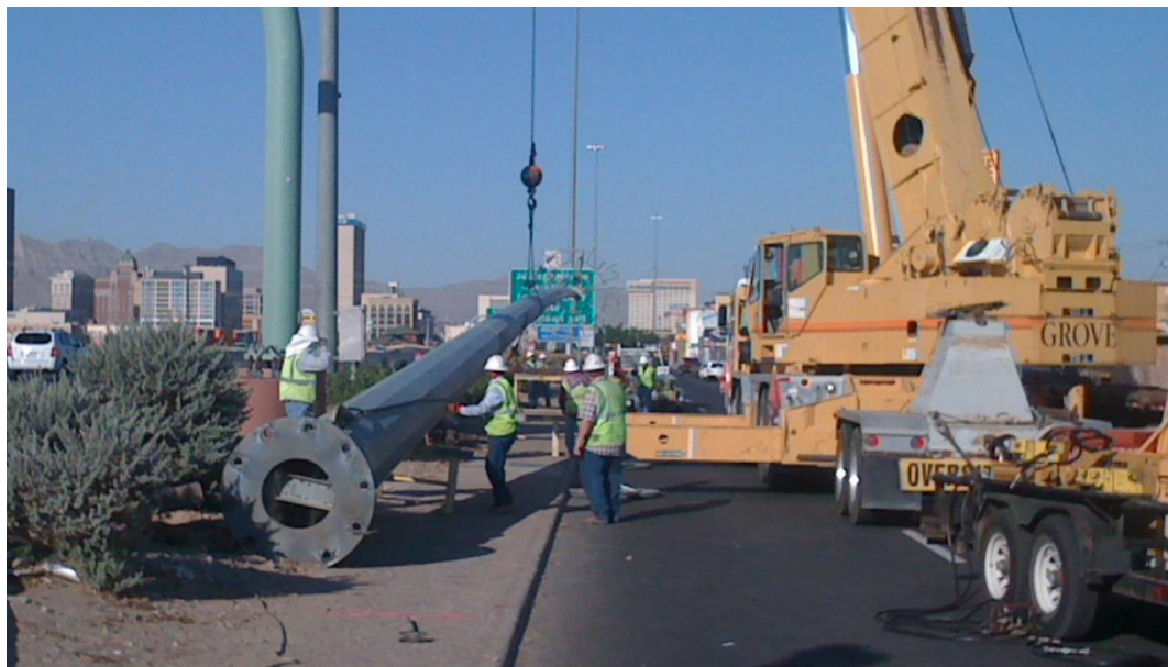
Figure 1.3: HMIP taken out of service
