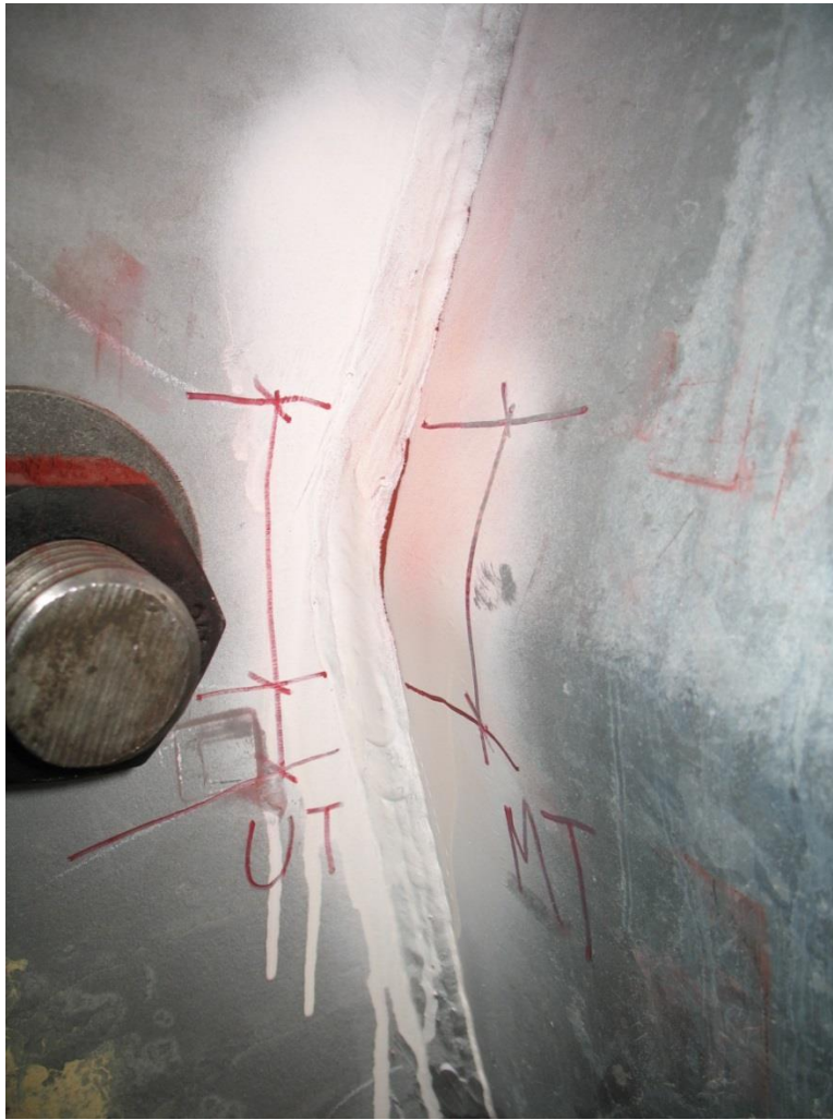
Figure 4.18: Crack location and width using MT and UT
