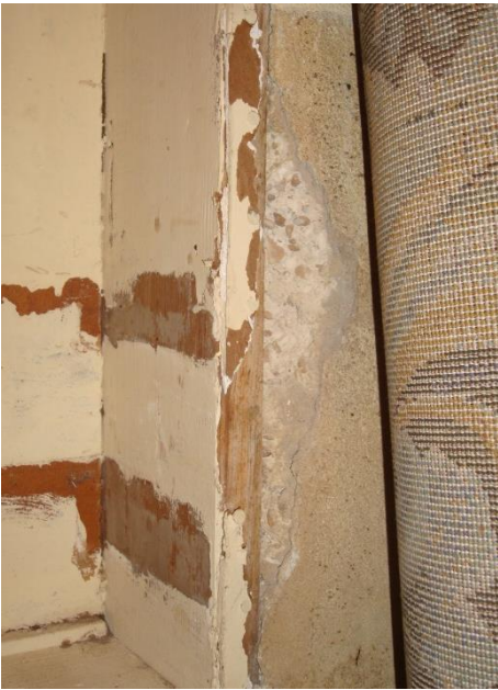
Figure 4.2: Window frame & exposed concrete, Author's image, September 12, 2013. The photo shows the small exposed area adjacent to the window frame that allowed for sample extraction.
