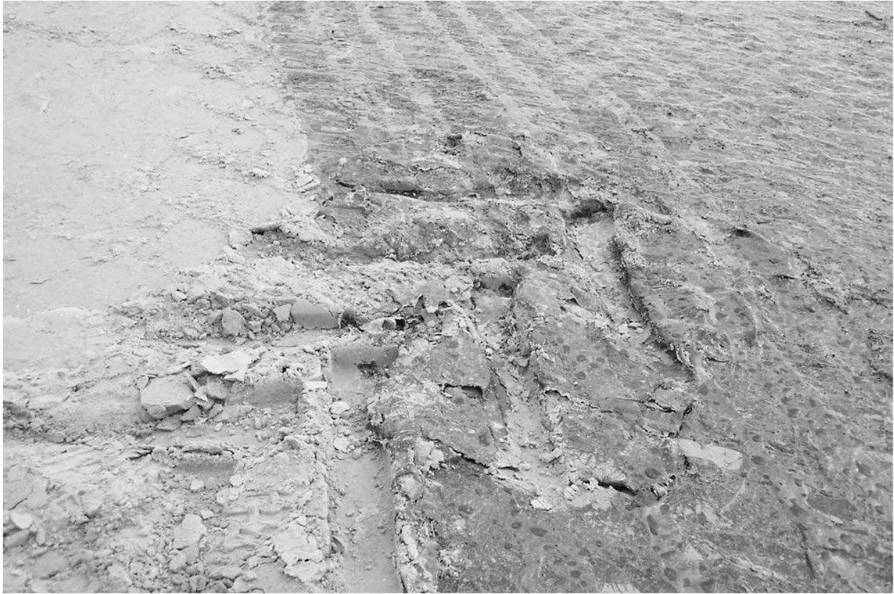
Figure 2.1 Emulsified asphalt with insufficient penetration (Cross, Voth, Shrestha 2005)
