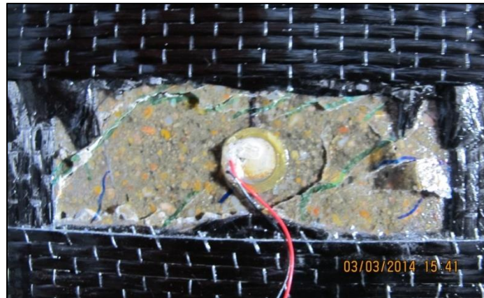
Figure 4-30: Cracking at the boundaries between concrete and CFRP
