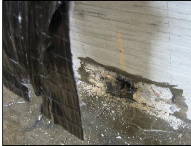
Figure 2-10: Anchor rupture observed when using the first detail (Quinn 2009)
