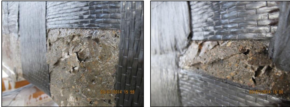
Figure 4-43: Development of cracks at CFRP edges for 14-3-Bi-D
