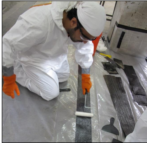
Figure 3-50: Impregnating both sides of CFRP strip before attaching it to the surface
