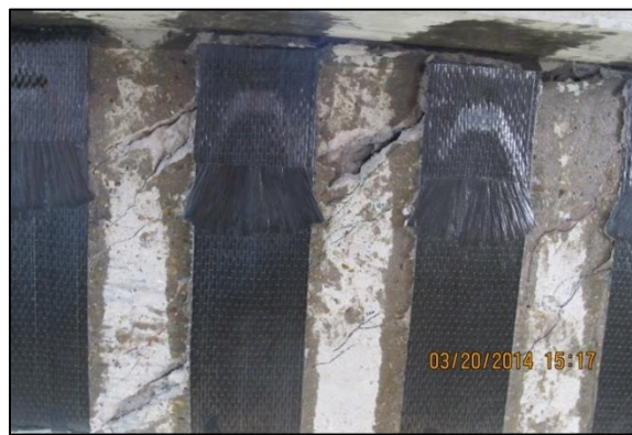
Figure 4-70: failure mode of 8-3-Uni
