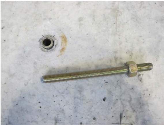
c) steel fracture
