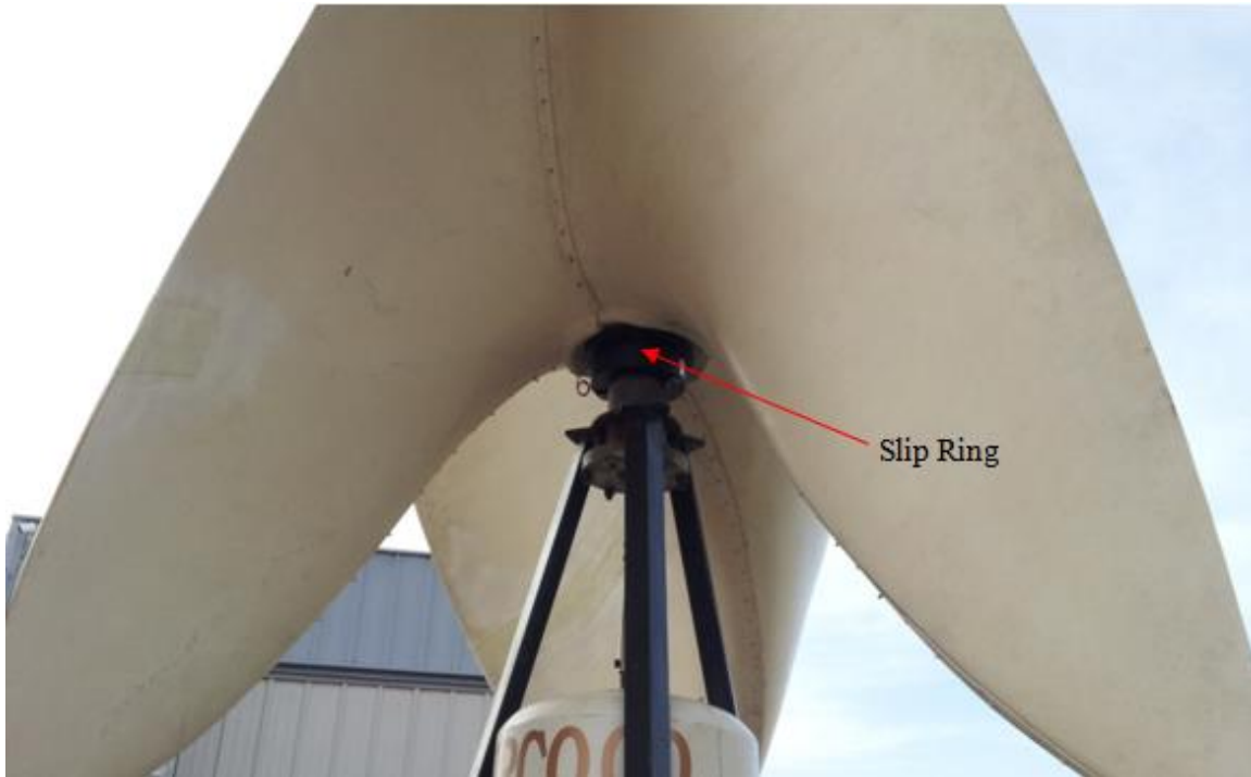
Figure 3.12: Close up view of the Marilyn turbine showing the Senring slip ring installed
