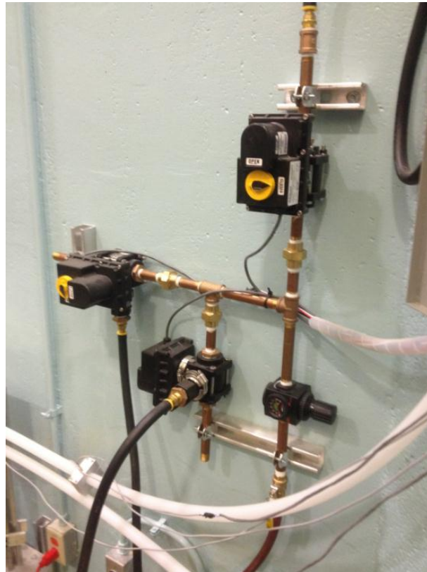
Figure 2.6: The manifold and valve assembly. The major components pictured are the three valves (left, top, and center), a dial pressure gauge (right), and a manual emergency cut-off valve (bottom right).
