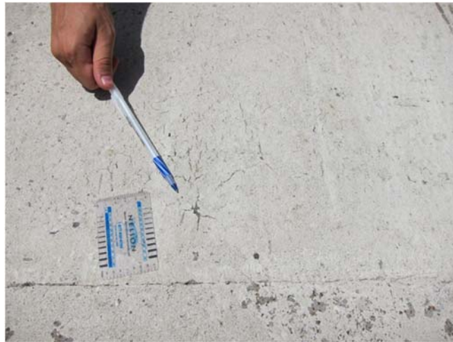
Figure 90: Plastic Cracking for CSA-1 Mixture at Cotulla Site
