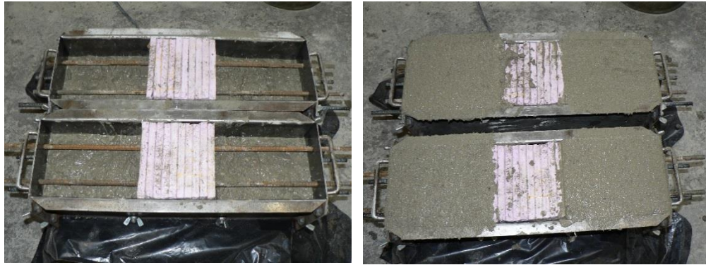
Figure 54. Casting top layer of fatigue-corrosion beams and displaying foam inserts for eventual repair material casting.
