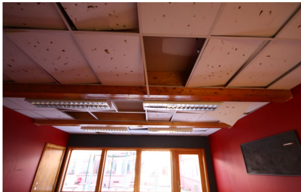
Damaged ceiling in the youth club reveals the glulam beams.
