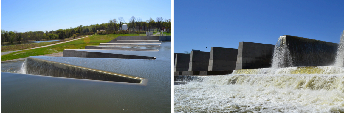
Fig. 13. Staged labyrinth spillway at Lake Townsend, Greensboro, NC, USA (Photo taken by Brian Crookston)
