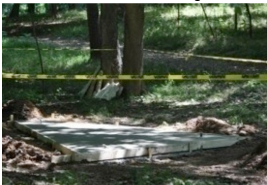
Integrated Concrete Pad/Piers
