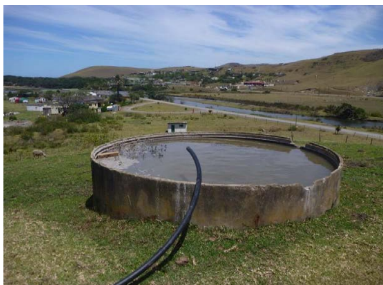
Figure 4.10: Pond overflowing from septic tank in Coffee Bay
