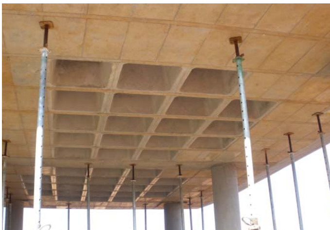
Figure 10.9 ~ DBSA coffer slab.jpg The roof structure, a reinforced concrete coffer slab. Source: HolmJordaan
