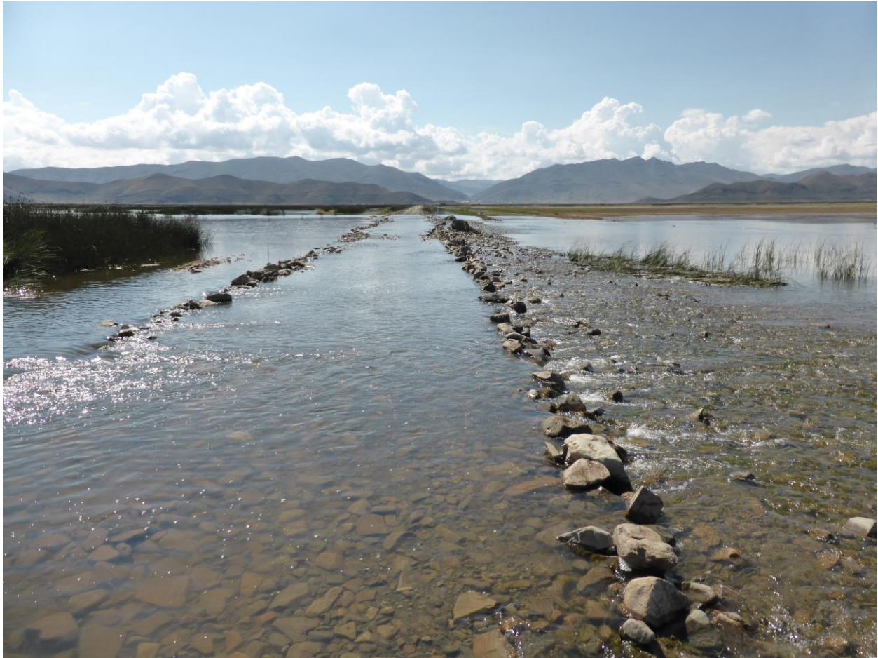
Figure 2: Washed out road to Poopó
