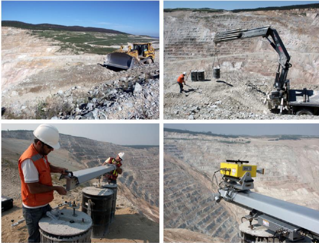
Figure 3.6. Site preparation and installation of the IBIS-M radar unit for the 3-D radar experiment, showing: leveling and grading of gravel site pad, lifting of concrete filled drums for radar base, fitting of leveled radar guide rail, and radar positioning for pit wall monitoring.
